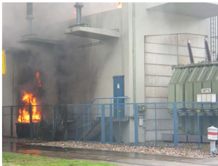
Figure 10. Flames and smoke occurring at the 2007 generator transformer fire at a German NPP
