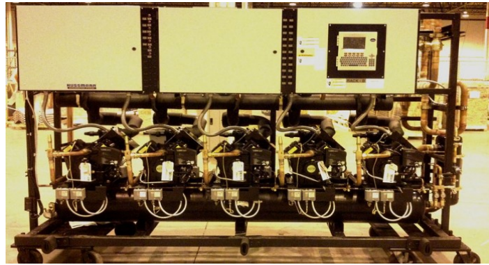
Figure 1: Parallel compressor Rack
