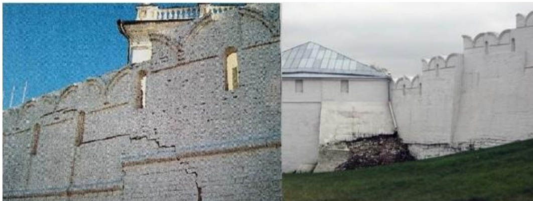
Figure 1: Deformations of the walls of the Kazan Kremlin (photo by the authors)
