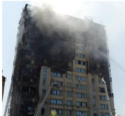
Fig. 1: Facade system with a ventilated air gap of a residential building after a fire, Baku, next to Azadlig metro station, 2015
